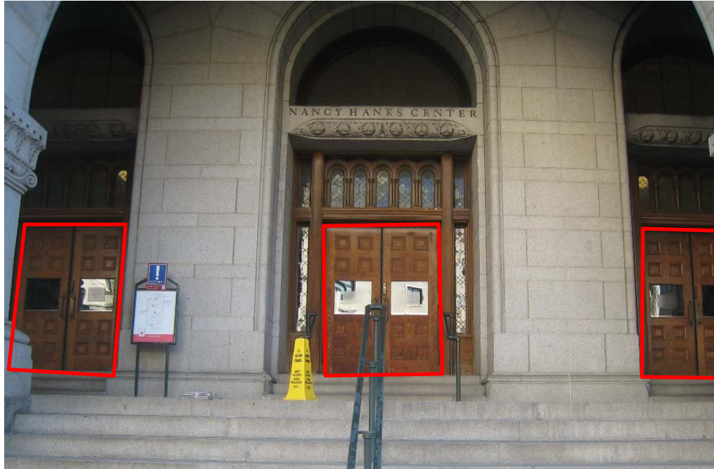
Existing wood door to be referbished.
